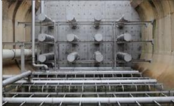
Figure 8. Aeration grids in the bottom of an MBBR reactor supply the oxygen needed for biomass growth
